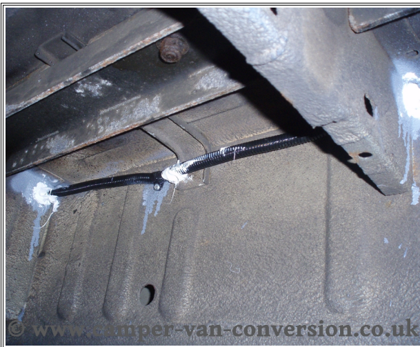
Secured cable (with cable shield fitted) under the van.
